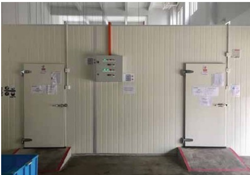
Walk In Chiller ( 0 - 4°C ) x 2 rooms
